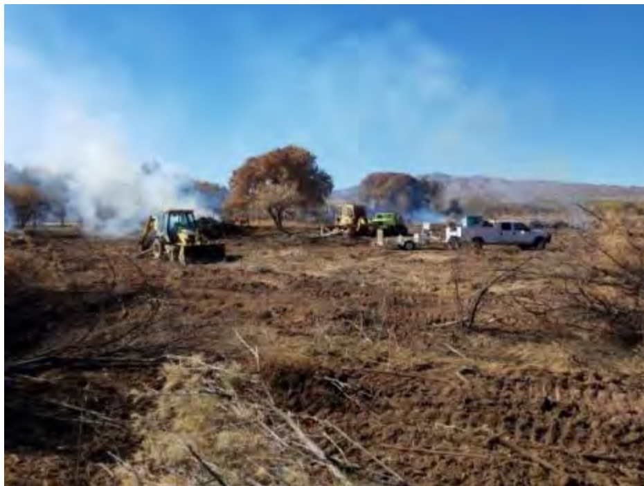
Clearing and burning work is underway in this picture. Native trees are left in place.
