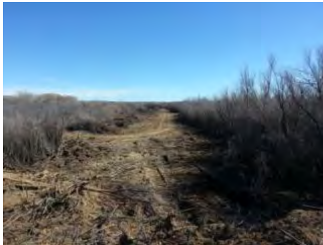
The contractor used Socorro SWCD supplied GPS technology to begin by clearing the property boundaries.
