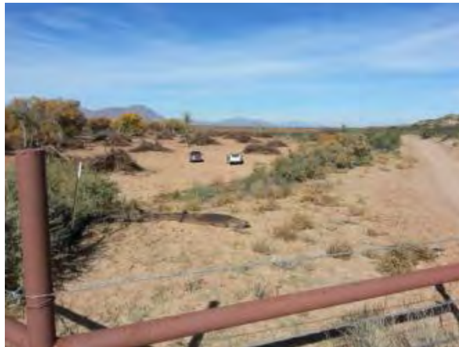
Rhodes property south, clearing and piling in progress. Bosquecito Road is on the right.
